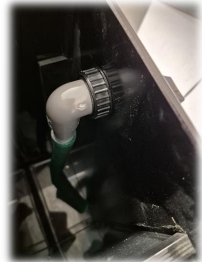
INTERNAL FILTERED WATER BULKHEAD W/ RETURN FITTINGS INSTALLED
